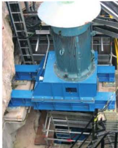
Figure 1 – Overhead view of seawater pump, one of four used in Borealis' ethylene plant
