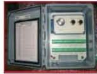
Figure 3 - Junction box showing selector switch for connection of accelerometer signals to PDC
