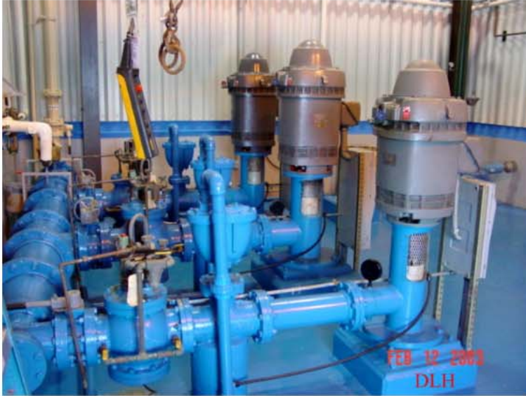
Figure 2. Vertical turbine pumps in clear well.
